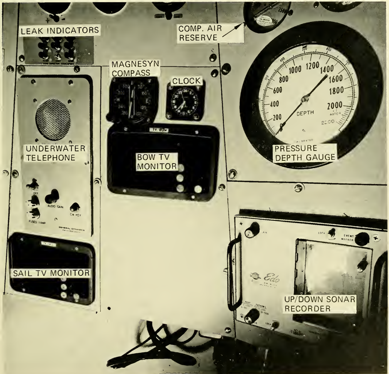
Fig 10.13 Various indicators and equipments aboard STAR III. (Gen. Dyn. Corp.)
